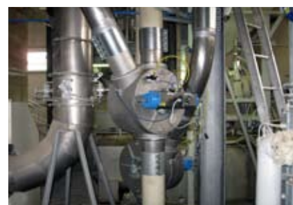
Drum-type diverter valve in pneumatic conveying system
